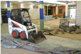
ABOVE ▲ "We had to rent a Bobcat and make a special blade with a lip to get under the carpet. Even then, removing the carpet was slow going," says Vasquez Jr.
